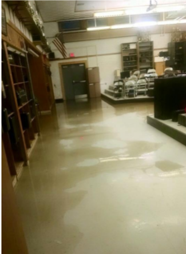
Figure 1: Because the State High band room is the lowest geographical point in State College, it floods nearly every time it rains, causing water damage to the building, storage, and instruments. Photo credits: Hannah Fecko
