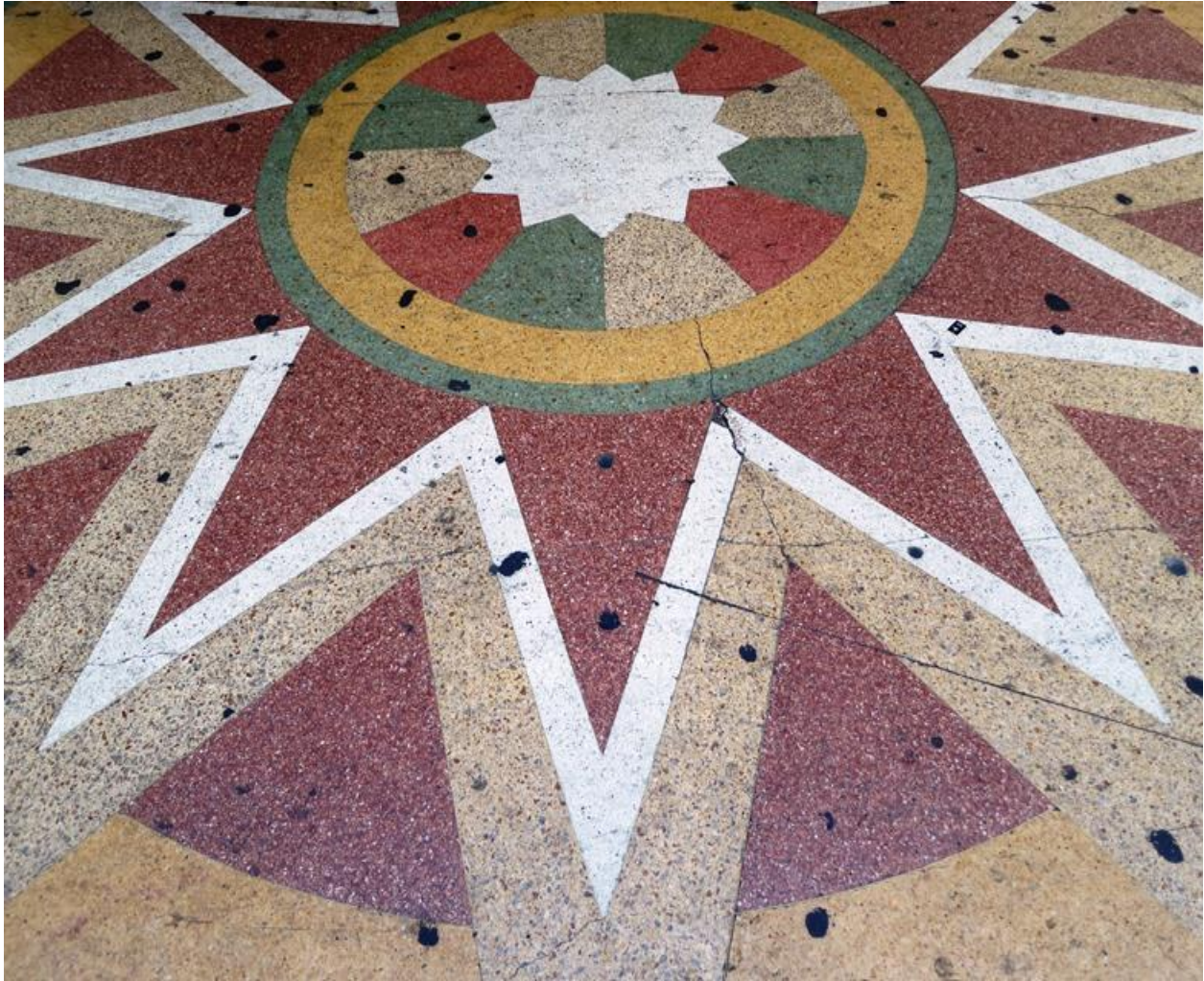
Figure 4.9. Detail of terrazzo tile in front of 648 South Broadway, with high artistic quality. Photo by author.
