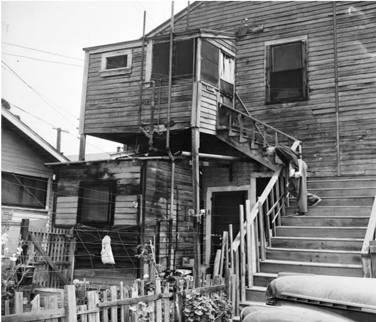
Figure 1.1. City inspector evaluates slum-like conditions in Los Angeles. Source: USC Libraries, Los Angeles Examiner Collection, File Name: EXM-N-9626-001~11.tiff.
