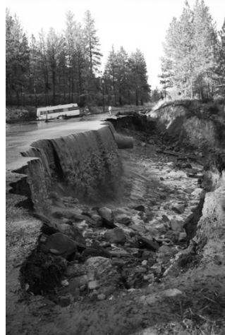
Flash flood & washout, Carlton complex fire: Washington Department of Transportation
