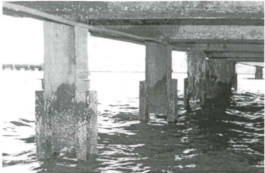
Fig. 4. Complete corrosion of steel H piles supporting a harbor pier. Note that recently installed retrofit channels are already corroding.
