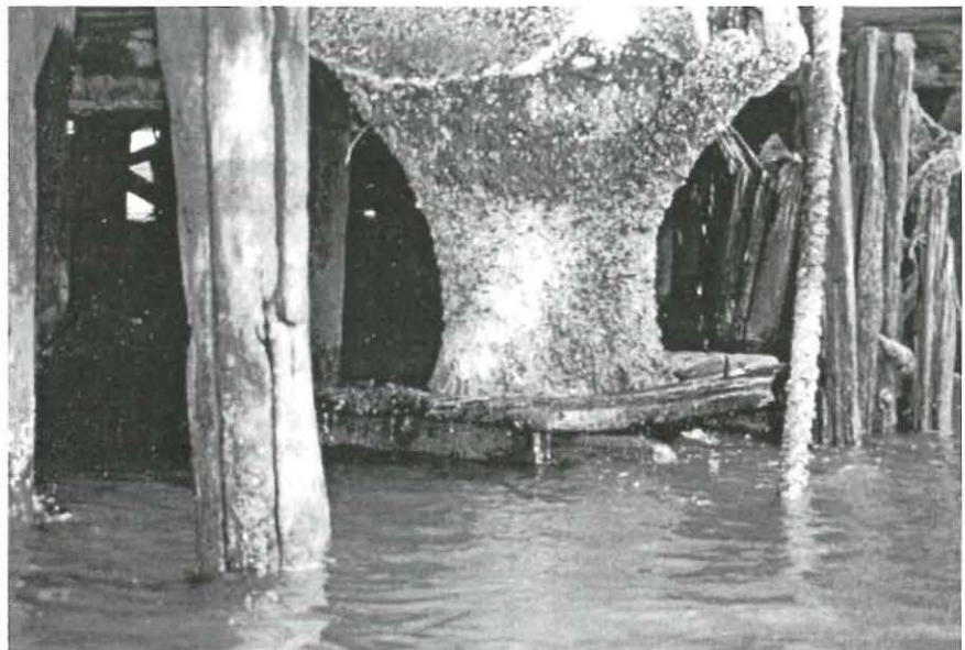
Figure 5. Deterioration of reinforced concrete piling supporting a harbor pier, causing it to lose 65% of its cross sectional area.
