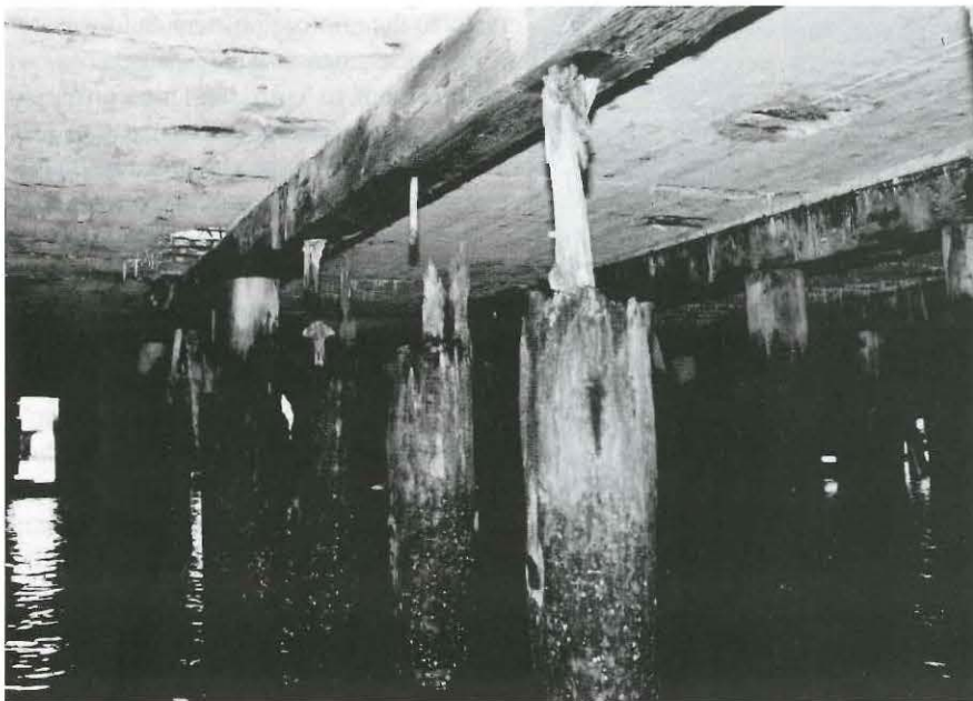
Figure 1. Marine borers (Limnoria) attacking untreated timber piles which support many of New York's pile supported highways and harbor piers.
