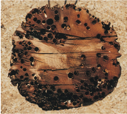
Figure 2. Limnoria Attacks on the Exterior of Timber Piling (top). Ship Worms (Teredo and Bankia) Tunneling Through the Interior of a Timber pile (bottom)
