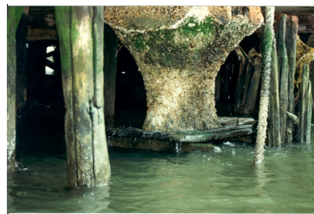
Figure 1. Complete Corrosion of Steel H Pile (top) & Loss of 65% of Cross Section of Concrete Pile (bottom)
